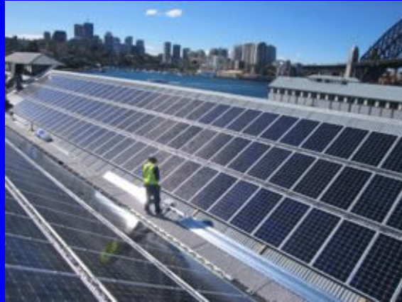
Wharf Theatre, Sydney, 384 kW
